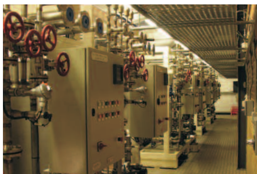
New extraction kicker oil cooling systems.
