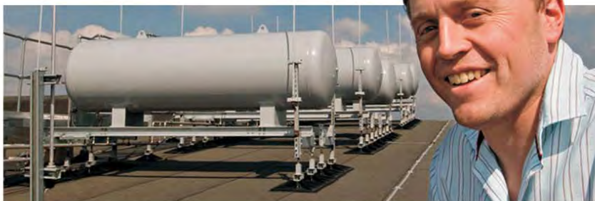
▲ Mike Ruddle (ISIS) in front of new buffer tanks for the first target station cryogenic moderators. Each has a capacity of 2000 l. Five are used to hold methane following the daily transfer, with the sixth for any gas vented from the hydrogen system. 09EC2030
